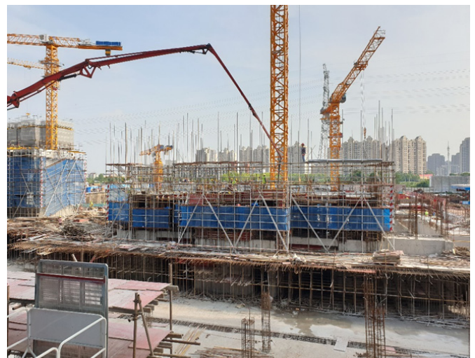
Construction Site for the 2nd phase of Shimao's Honor of China project
